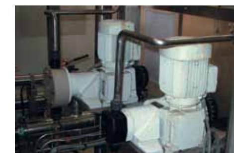
Metering of soda and acid.
