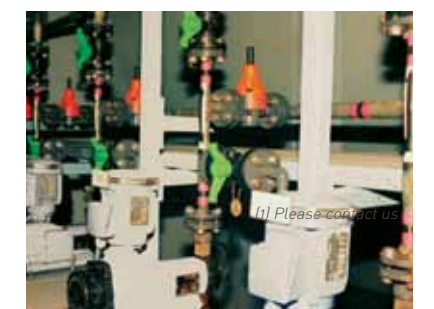
Ferric chloride pumping in purification station.
