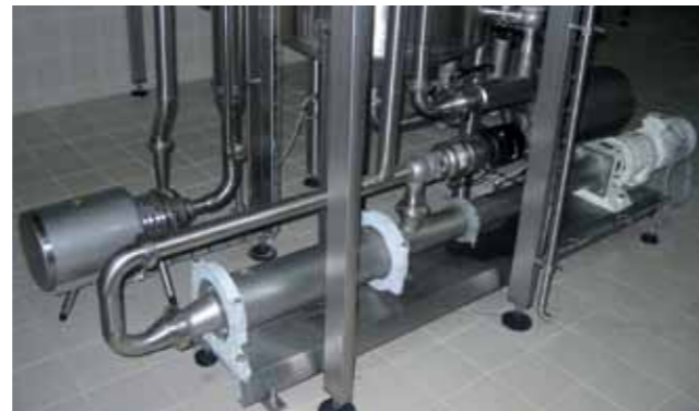
PCM pump in dairy application
